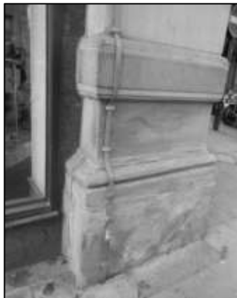
Figure 19: Sandstone in Manchester city centre. Spalling probably caused by salt damage.
