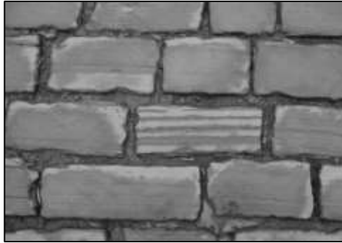
Figure 18: Weathered sandstone setts in Lancaster city centre, showing splitting along micaceous partings.
